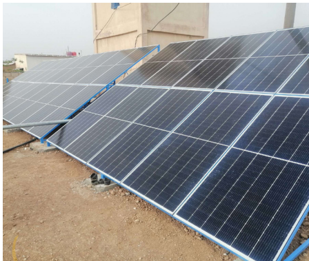
Solar panels installed by Acted in Ar-Raqqa, Syria
